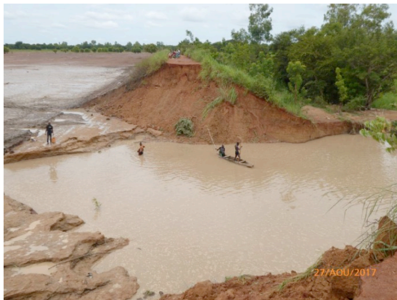
Figure 14: Broken dam of Koubri after heavy rainfall August 2017 (Source: R. Ouédraogo)
